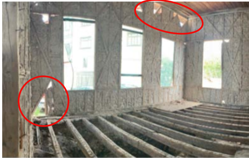
Image 2.6: Safranbolu, used to be an old house, its waiting to be restored into an elementary school.
